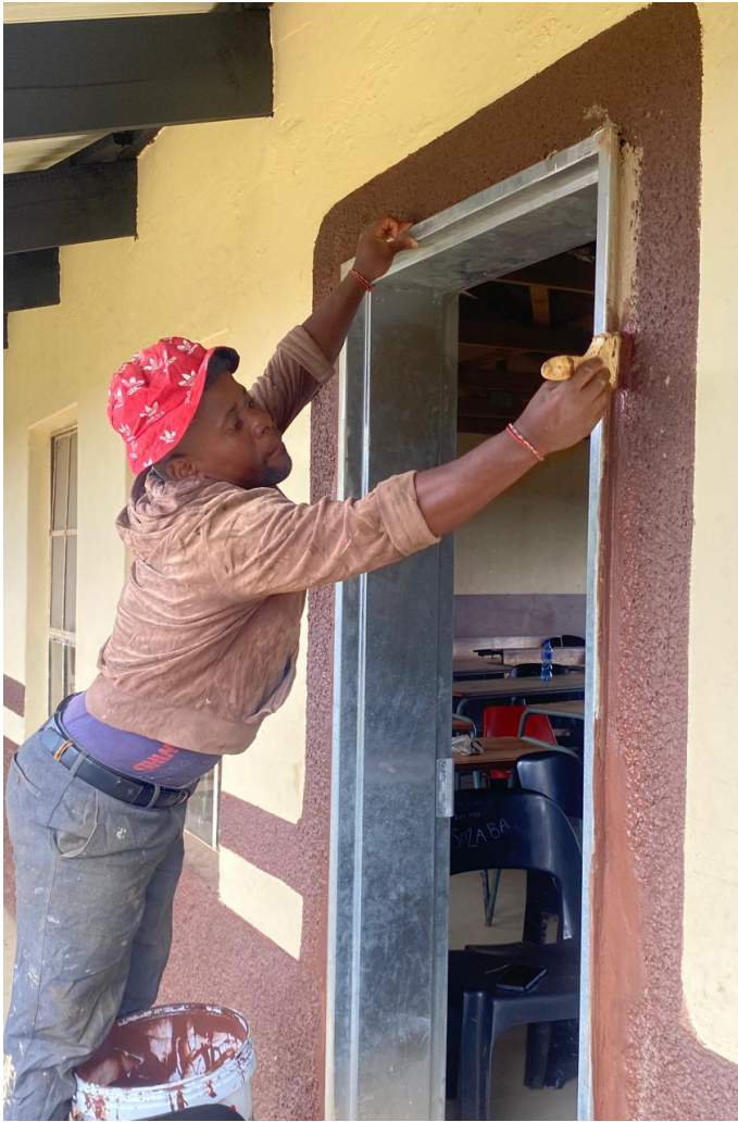
The Hlokozi PRC carried out renovation work on Luswazi Secondary School to improve conditions for learners.
